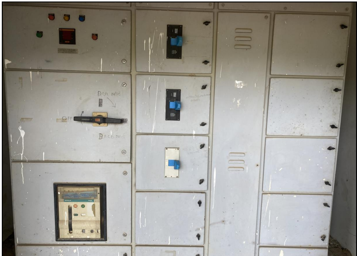
Figure 2.5 Capacitor bank on main panel
