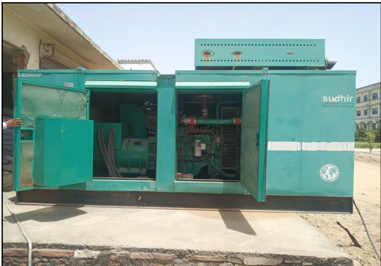
Figure 2.4:- DG set in Power House
