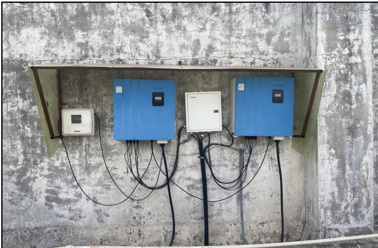
Figure 2.6:- Solar Plant 480 KWp and Inverter System
